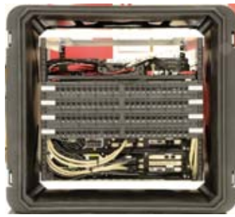
Rack Open—Demarcation Panel
